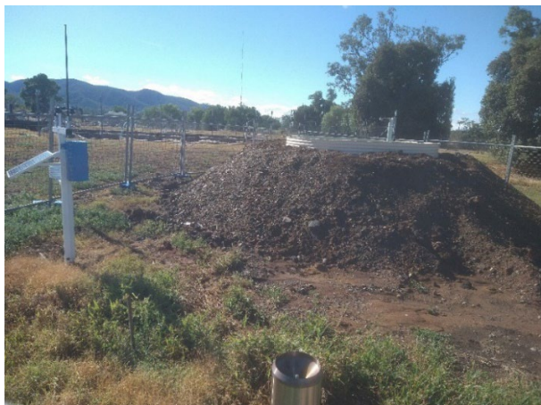
Figure 9 Initial brine tank installation December 2023 (in-ground 0.6m, 2.1 m above ground) showing dedicated weather station (left) and rain gauge (foreground)
