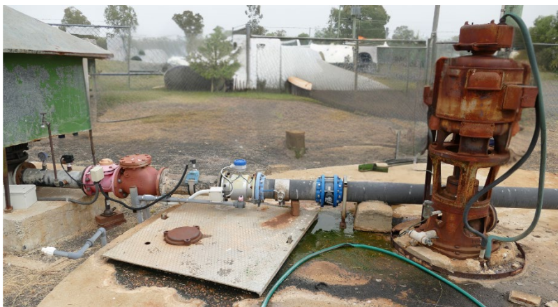
Figure 1: A drinking water bore from WSP in south-west Queensland, which is more than 100 years old. This bore provides backup drinking water supply.
