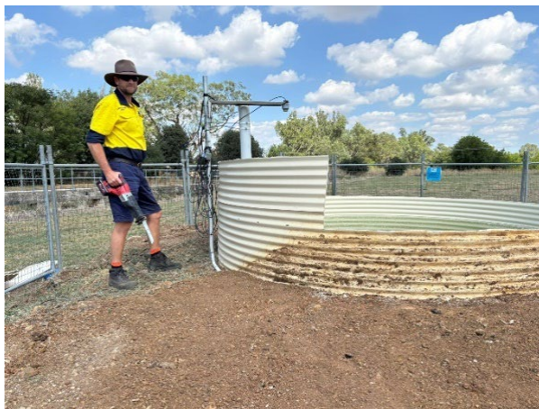
Figure 10 Second wall cut-down February 2025. Brine level visible inside tank, 300mm below new wall height.
